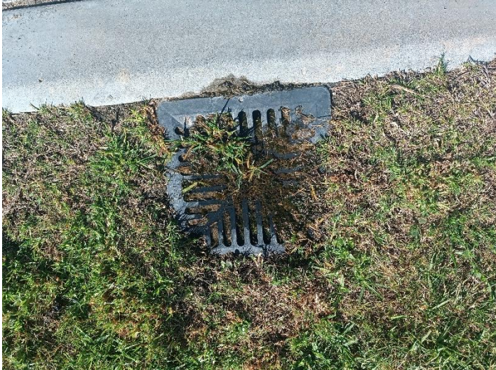
Figure 13: Storm water drain blocked by silt and vegetation offcuts
