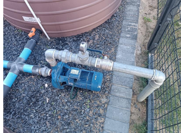
Figure 14: Borehole pump with no water use license
