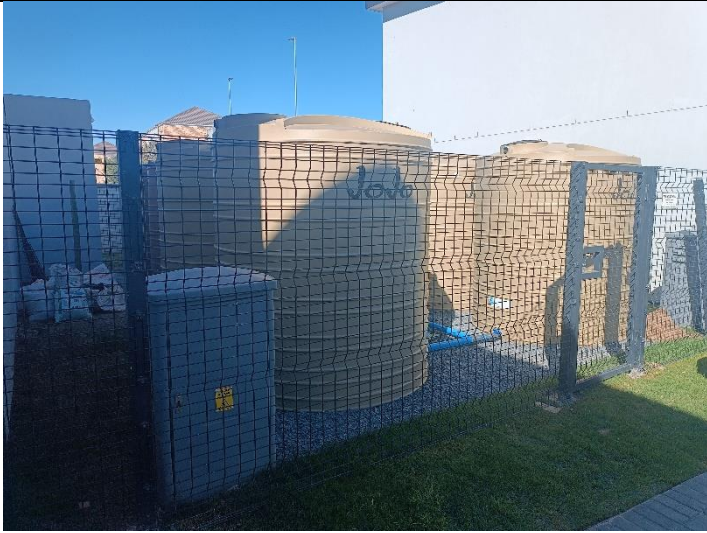
Figure 15: Water tanks for the borehole pump
